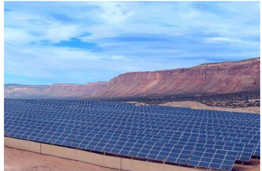
Paradox Community Solar Array in Naturita, Colorado (Courtesy of Clean Energy Collective)
