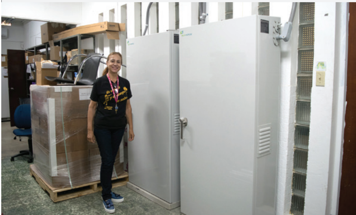
View of the 20-kW Sunverge battery storage system at the Clinica Profamilia in San Juan, Puerto Rico. This community medical clinic was the recipient of technical and financial support from CEG's Technical Assistance Fund, enabling the installation of a resilient solar+storage system.
