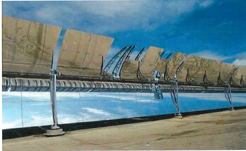
[http://d2r42o2f7hk334.cloudfront.net/wp-content/uploads/2012/08/genesis-flood-5.jpg] Damaged parabolic trough solar collector. (image via NextEra Energy)
