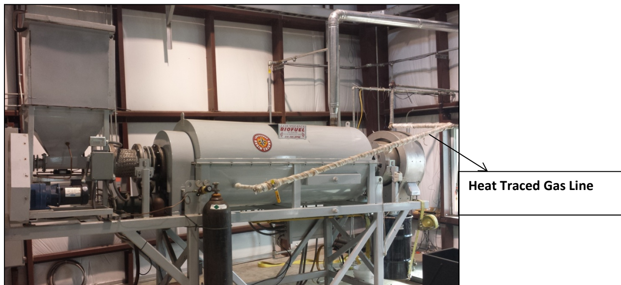
Figure 1: Torrefaction reactor retrofitted with heat traced gas line to route volatiles and gases into natural gas combustion zone.
