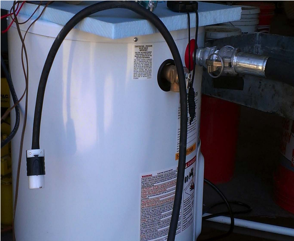
Figure 17: Heater to maintain digester temperature.
