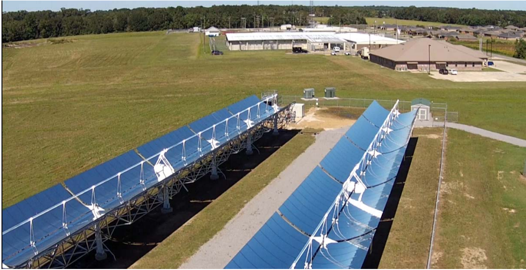
Figure 14: Aerial Photograph of Solar Thermal Power Plant While in Operation
