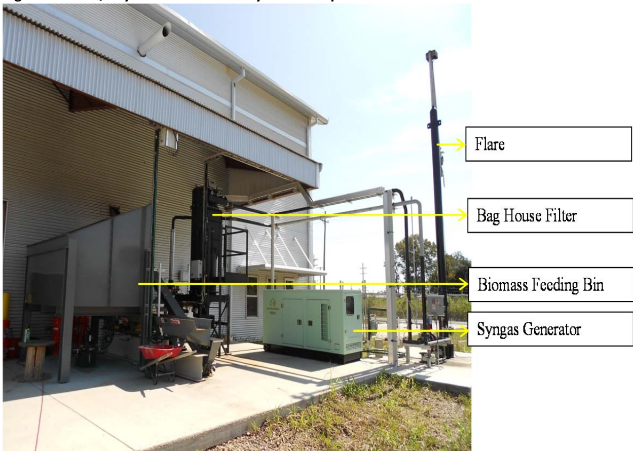
Figure 5: 3 ton/day BFB Gasification System Components
