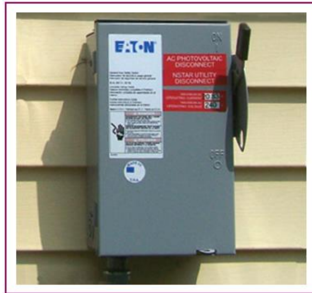
EXHIBIT 690.10 PV system disconnect.
