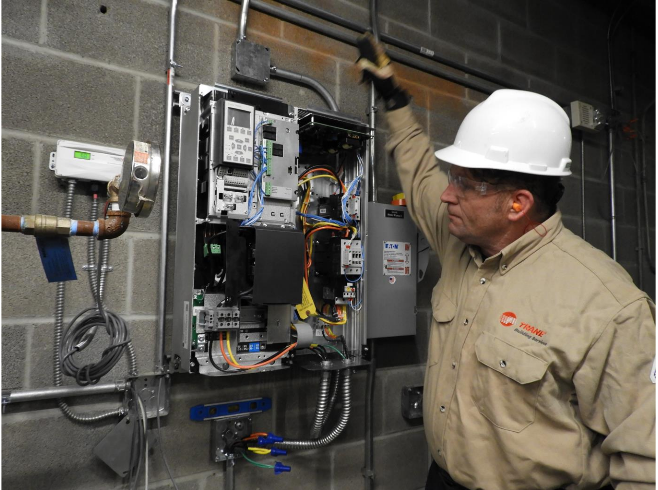
Custom Commercial project: Chiller/Controls/Variable Frequency Drive (VFD) upgrade project by registered trade ally, Trane.
