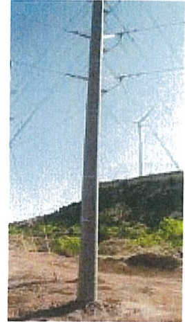
Figure 1: Composite Distribution Pole
