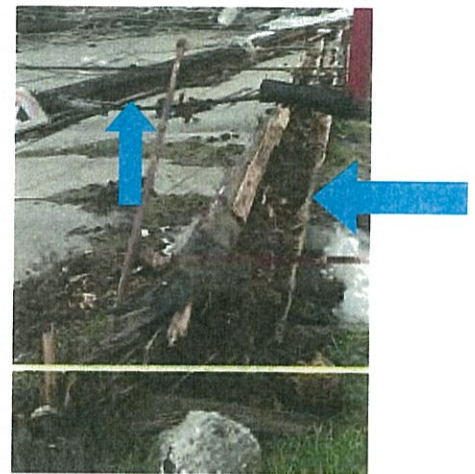
Figure 1: Fallen Wood Pole in New Orleans East After February 7 th , 2017 Tornado
